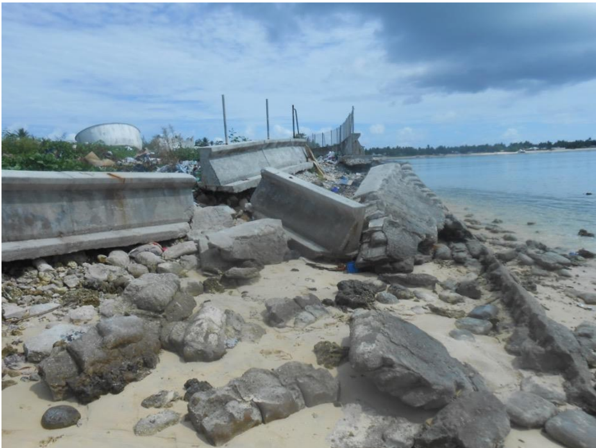
Photo 13: Betio dumpsite wall damage from wave action, July 2016
